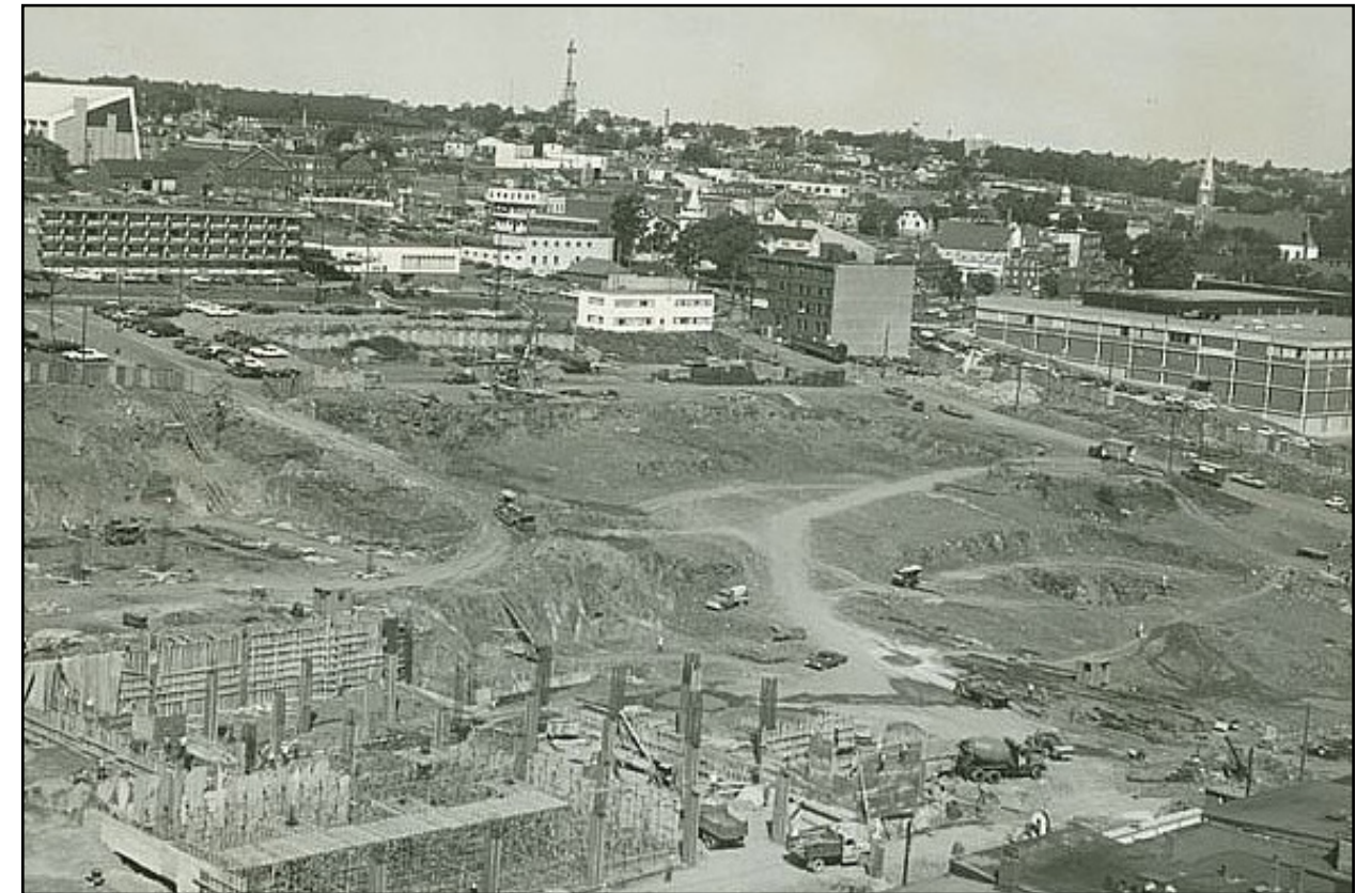
Urban renewal underway, 1967. Duke Tower excavation site looking north towards Gottingen Street. (NSARM, 1967).
