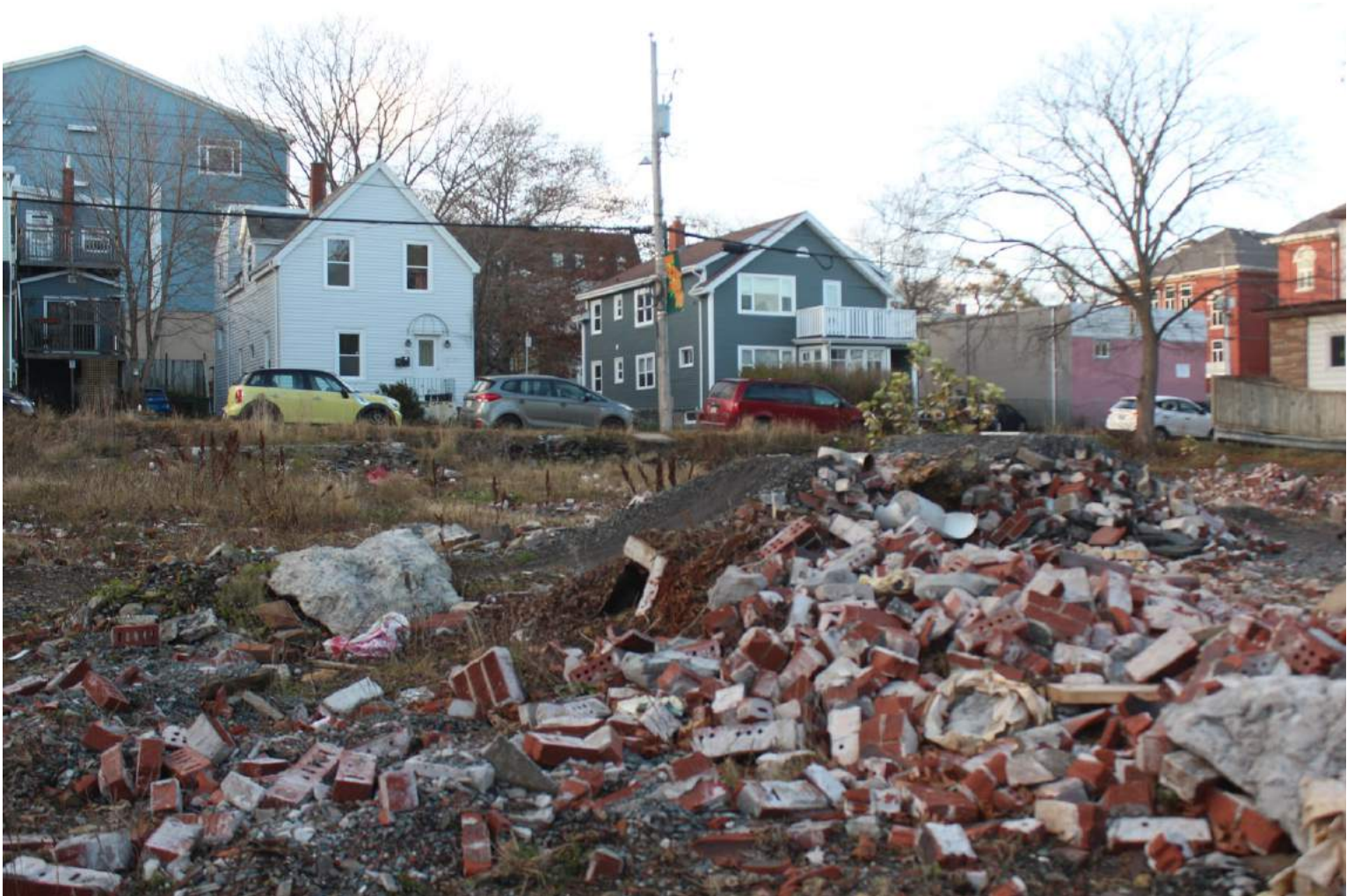
Demolition remains from former rooming house in Dartmouth, NS (Photograph taken by Uytæ Lee, 2016)
